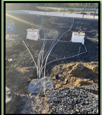
Underground Utilities from Monitoring Station
