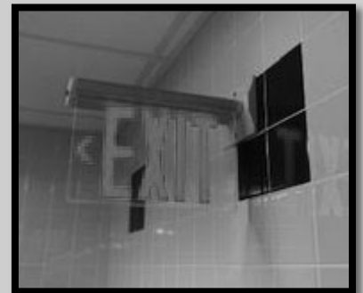
New Exit Lighting building wide in the High School
